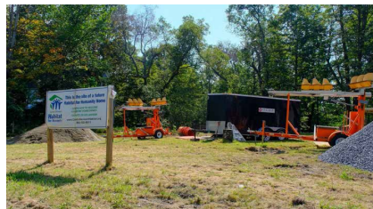
Initial work began this week on the future Habitat for Humanity home on Central Street. (Herald / Kyan Smith)
